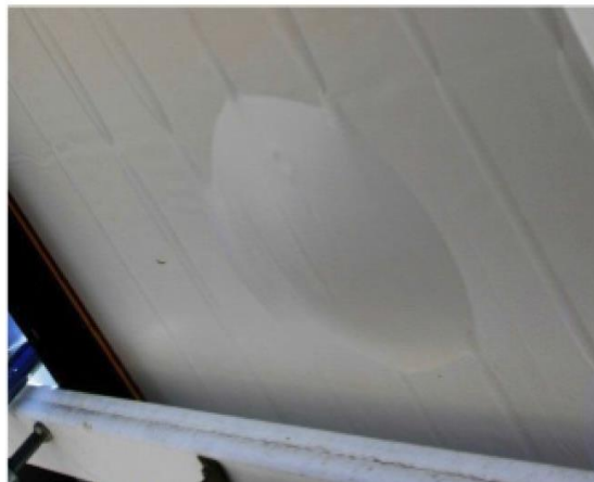
Figure 2.7. Delamination of backsheet [11]
