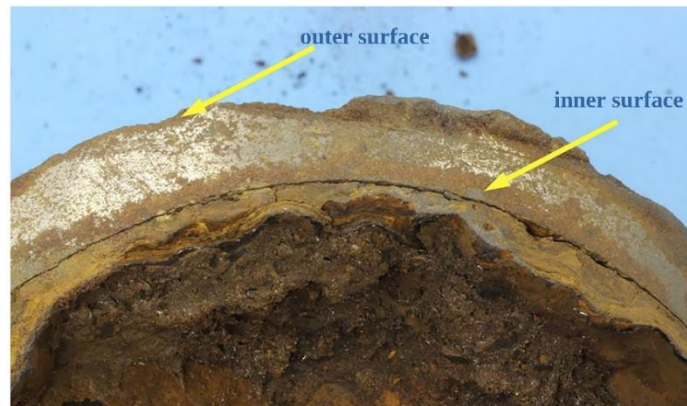
Figure 3. Closer view of pipe wall in cross section; arrows point to corrosive attack at inner and outer surfaces. Reprinted from ref. [21].
